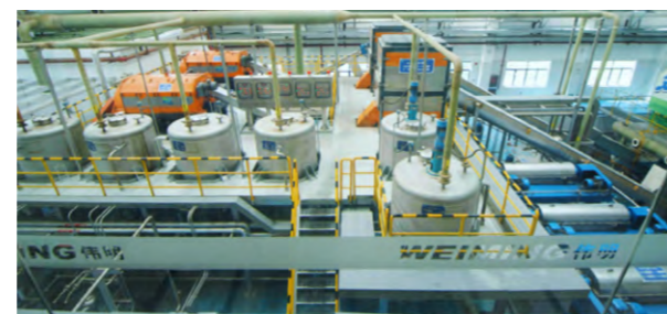
the workshop of kitchen waste treatment project
