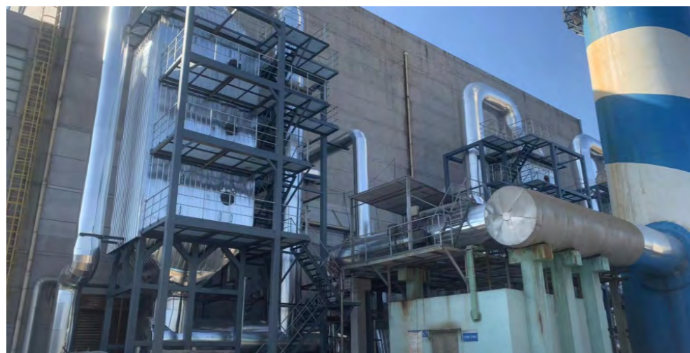
External denitrification equipment of Kunshan Project
